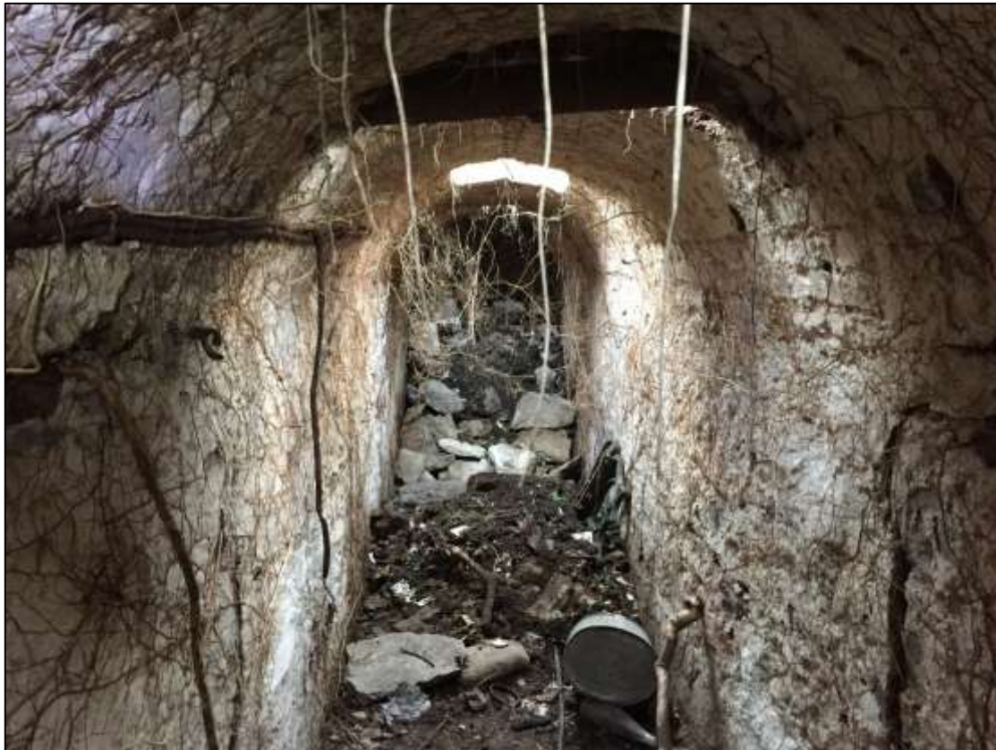
Plate 61. Debris closing western end of the service tunnel.
