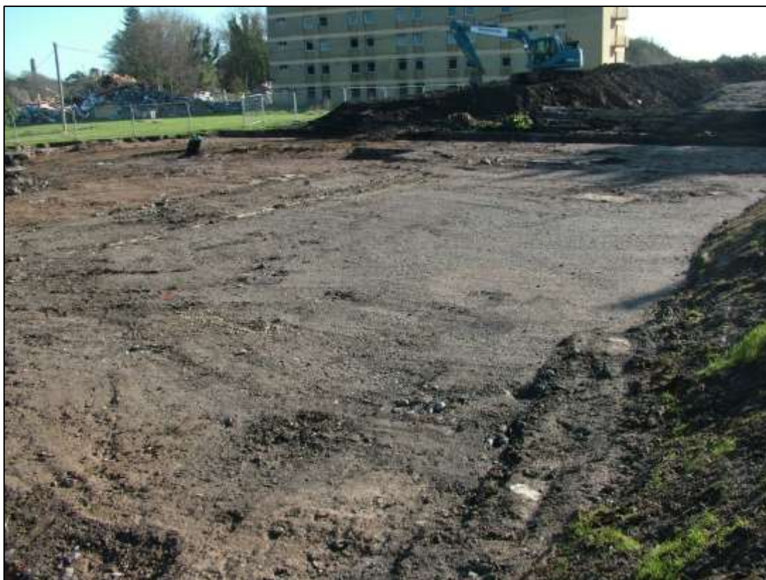
Plate 22. Area 1 – Yard surface looking SE. Nurses block to the S
