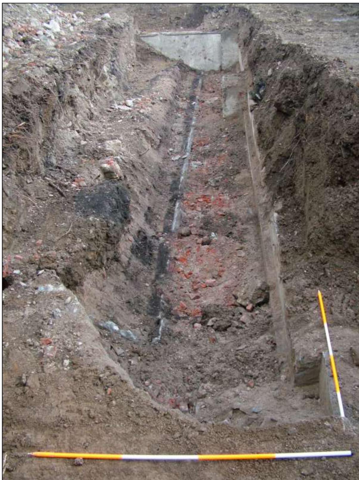
Plate 40. Area 3 – Excavation to reveal external wall face and drainage, Portrane House. Looking E
