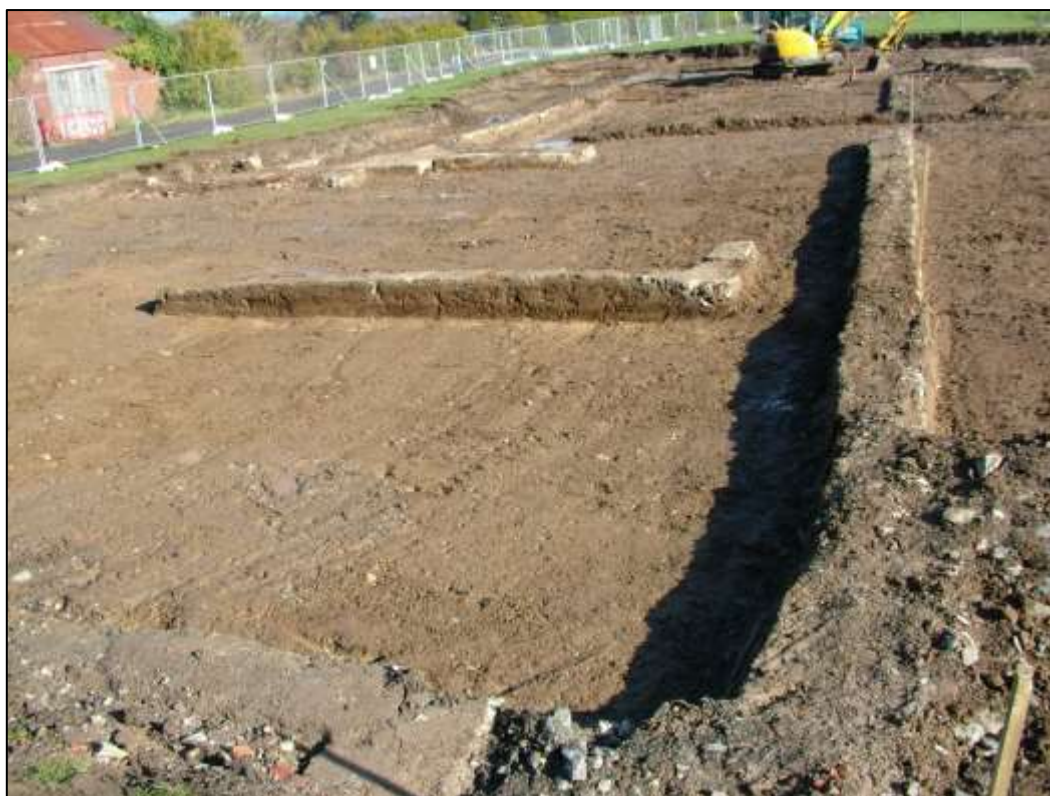
Plate 23. Area 1 – Temporary No 2 / Block 8/8a looking E over Scullery and Dining Room
