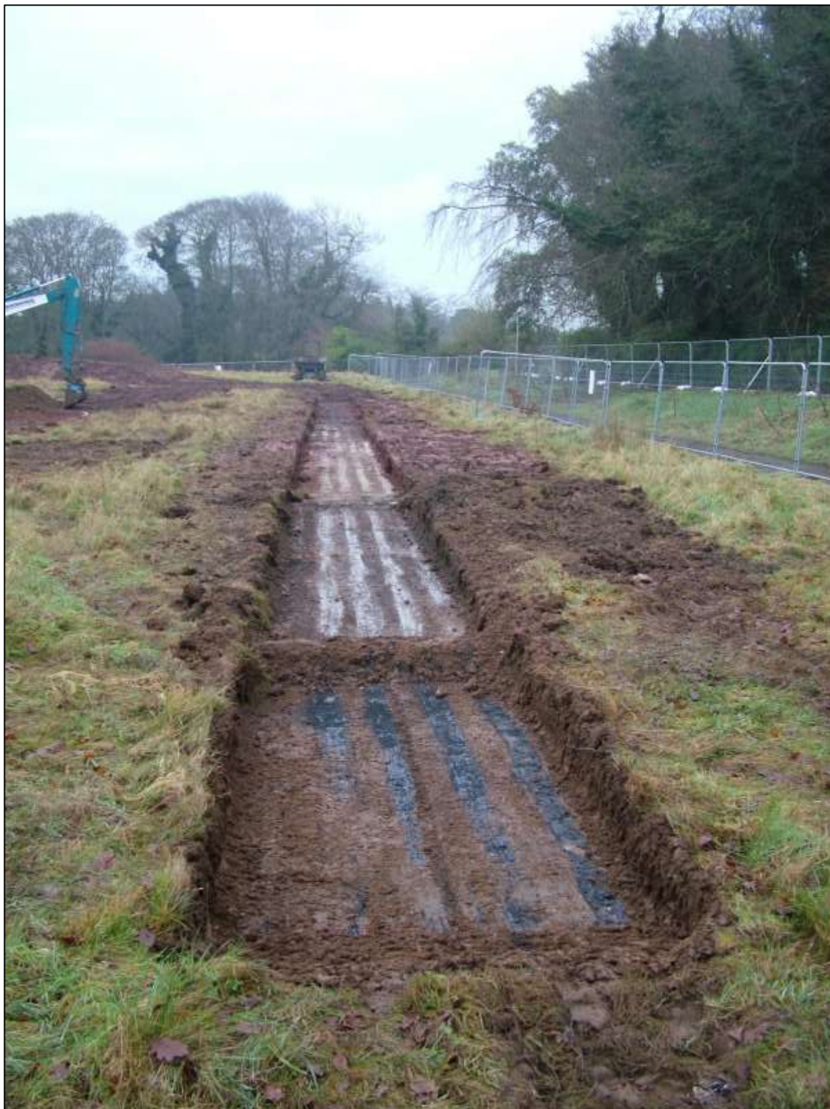
Plate 6. Area 2 - Stripping topsoil from Temporary No 4 / Block 9 looking east. Topsoil strip exposed the asphalt layer on which the floor boards were placed.
